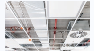
② Cable inlets, ducts, lighting fixtures
