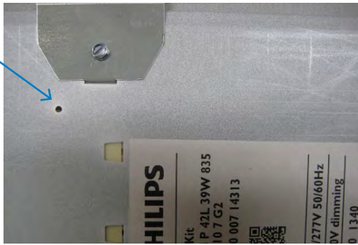
Picture C. Existing hole in LED Panel
